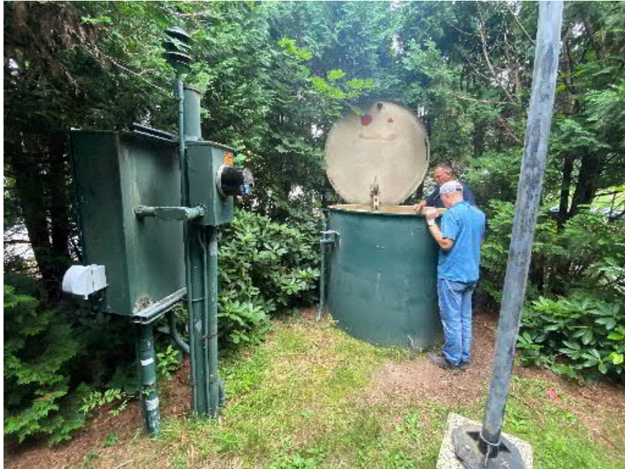
Topors Pump Station: Prefabricated Pneumatic Pump Station.
