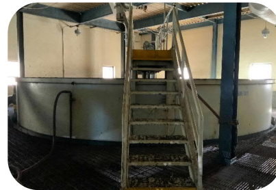
Gravity Thickeners and Sludge Collectors
