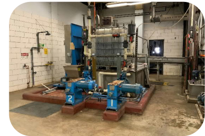
Polymer and Dewatering Equipment
