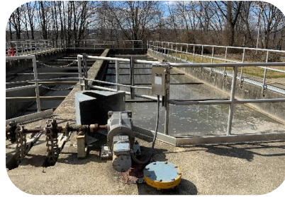
Primary Clarifier Sludge Collectors
