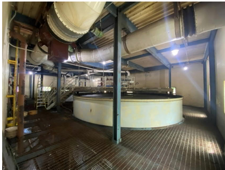
Operations Building 2 nd Floor: Gravity Thickener Tanks.
