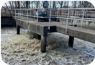
Mechanical Surface Aerators
