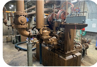
Primary Sludge Pumps
