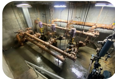
Return/Waste Activated Sludge & Scum Pumps
