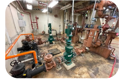
Primary Scum Pumps
