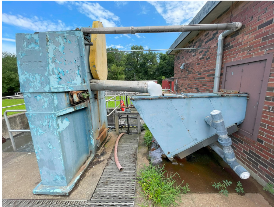
Aerated Grit Facility Equipment: Grit Elevator.
