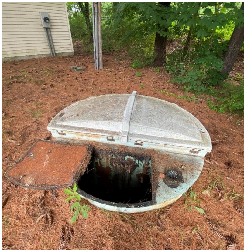
Morgan Street Pump Station: Wet Well Enclosure for Submersible Pumps.
