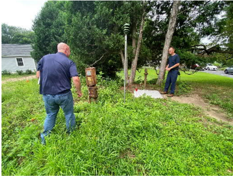
Old Sycamore Pump Station: Meter and prefabricated Pneumatic Pump Station Enclosure.
