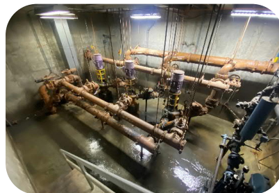
Return/Waste Activated Sludge & Scum Pumps
