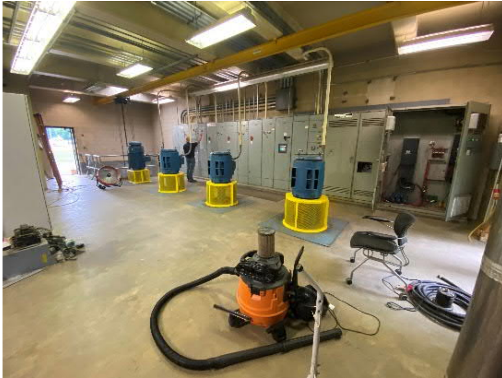
Main Street Pump Station 4 th Floor: Four (4) Vertical Dry Pit Pump Motors.
