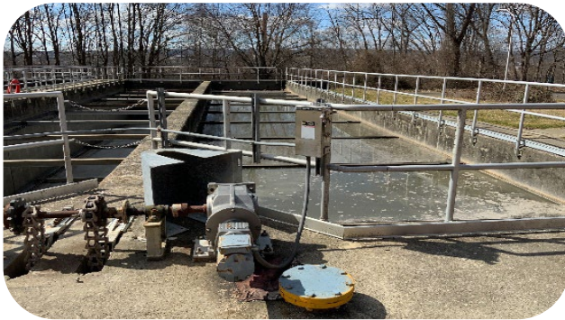
Primary Sludge Collectors
