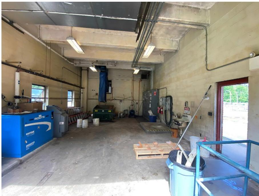
Grit Building: Grit Chamber Blowers (left), Grit Shute and Dumpster (center), Control Panel (right).
