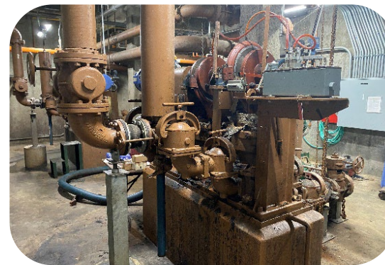
Primary Sludge Pumps
