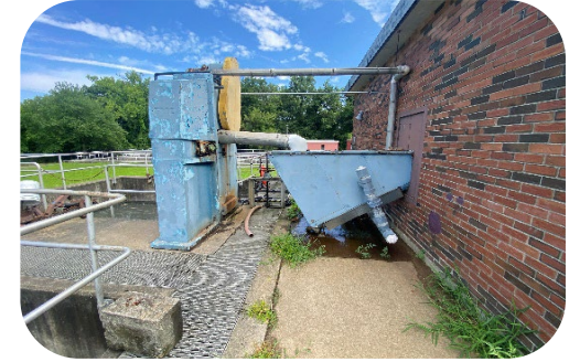
Grit Bucket Elevator
