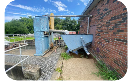
Grit Bucket Elevator
