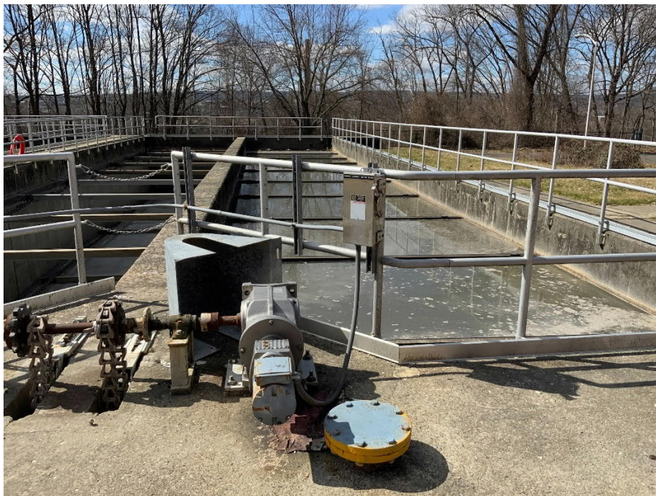
Primary Treatment Equipment: Primary Clarifiers #2 & #3 Drive Mechanism.
