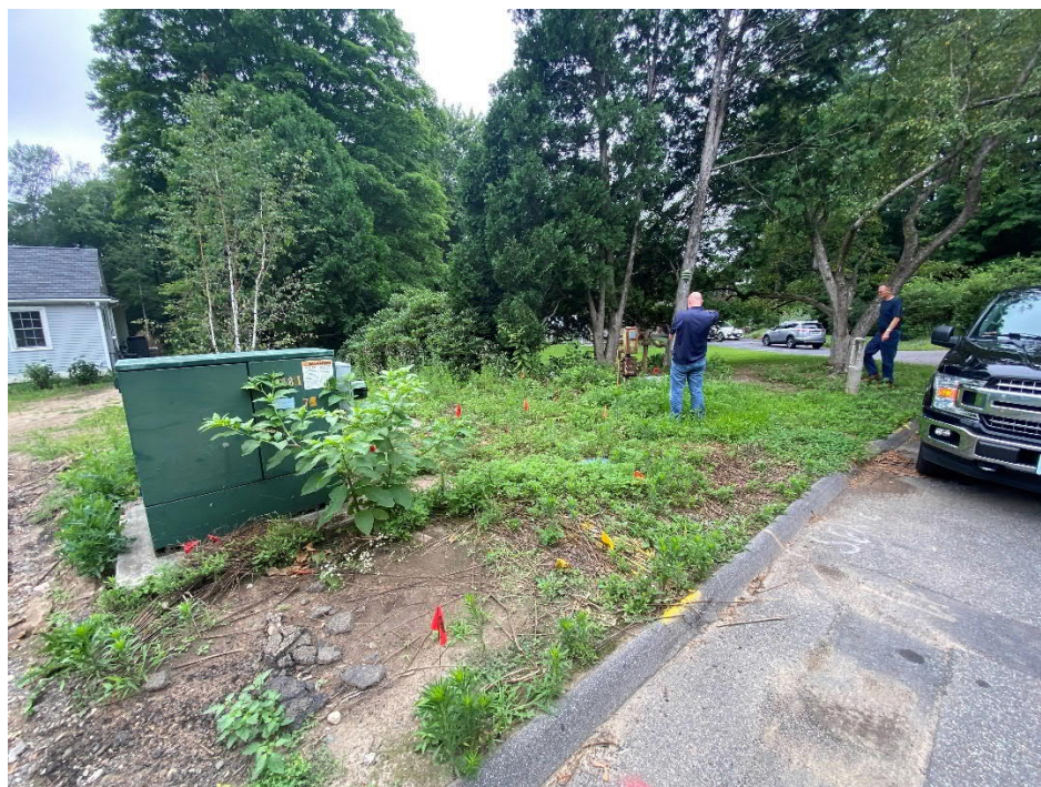
Old Sycamore Pump Station: Transformer.
