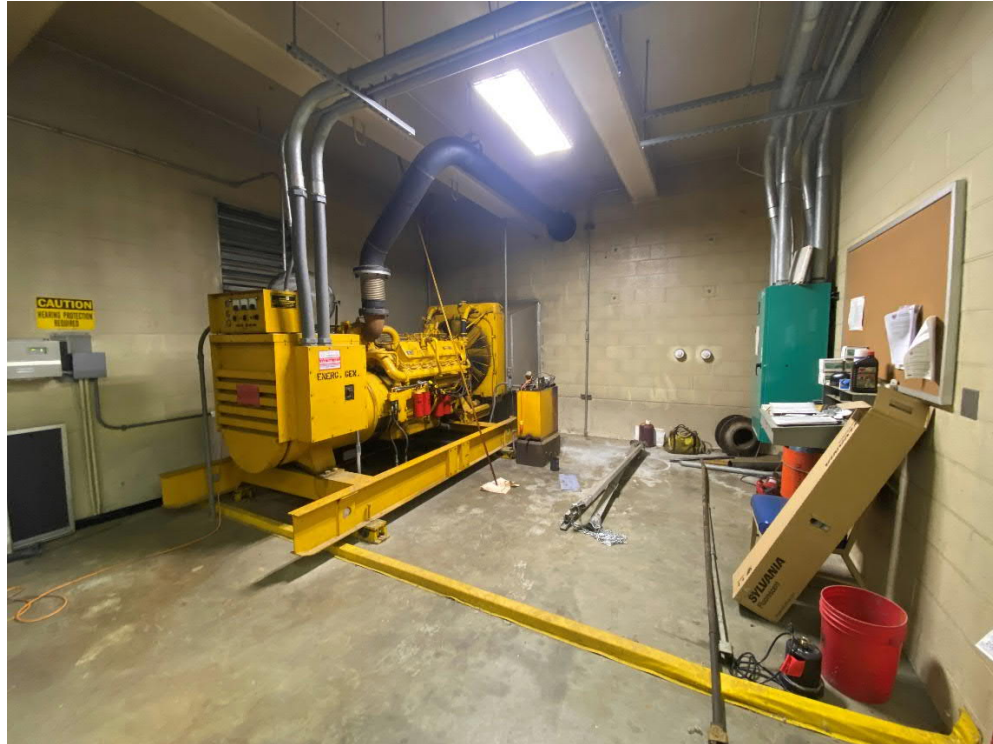
Main Street Pump Station 4 th Floor: Generator.
