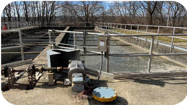
Primary Sludge Collectors
