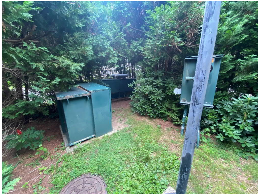
Topors Pump Station: Generator and transformer.
