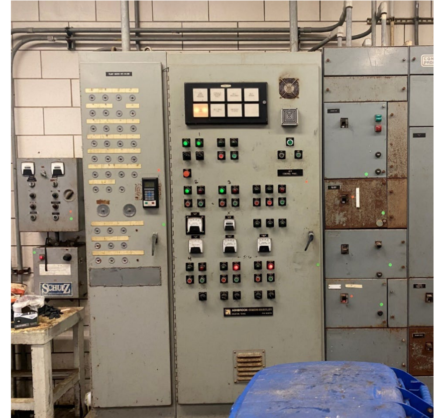
Typical Electrical Panel
