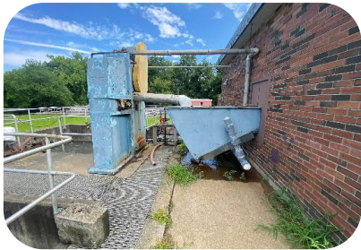
Gravity Bucket Elevator
