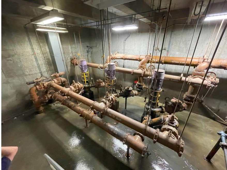
Return Sludge Pump Building: RAS Pumps.
