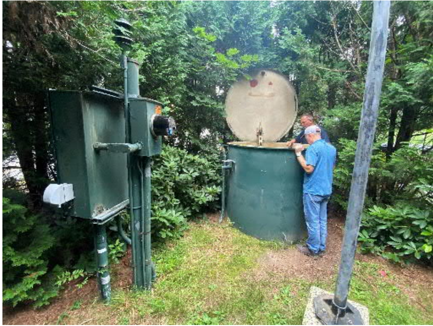
Topors Pump Station: Prefabricated Pneumatic Pump Station.
