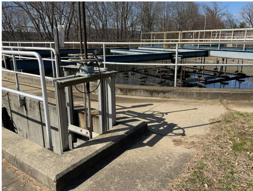
Secondary Clarifier: Secondary Clarifier #2 & Parshall Flume.
