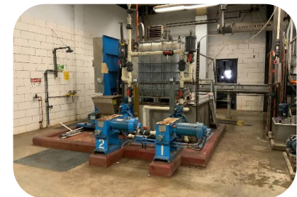
Polymer and Dewatering Equipment
