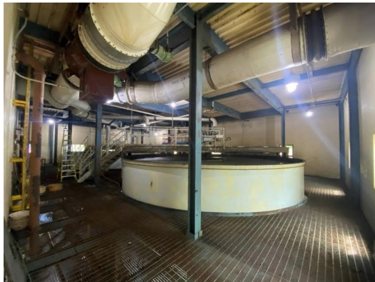
Operations Building 2 nd Floor: Gravity Thickener Tanks.
