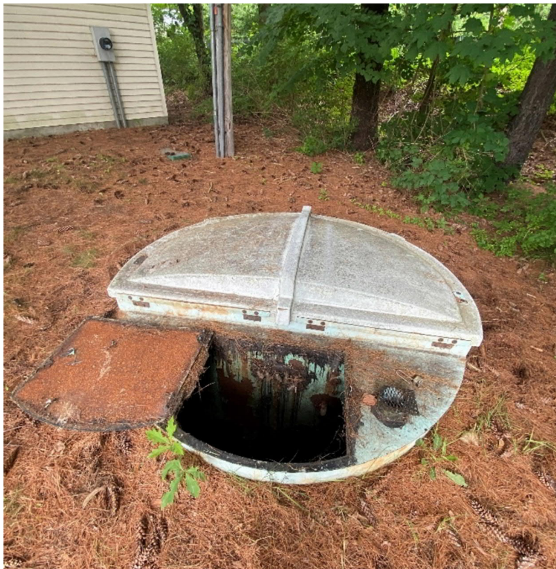
Morgan Street Pump Station: Wet Well Enclosure for Submersible Pumps.
