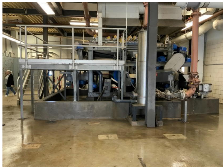
Operations Building 2 nd Floor: Belt Filter Press
