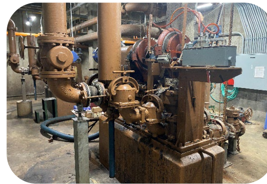
Primary Sludge Pumps
