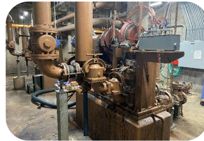
Primary Sludge Pumps
