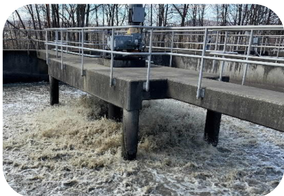
Mechanical Surface Aerators
