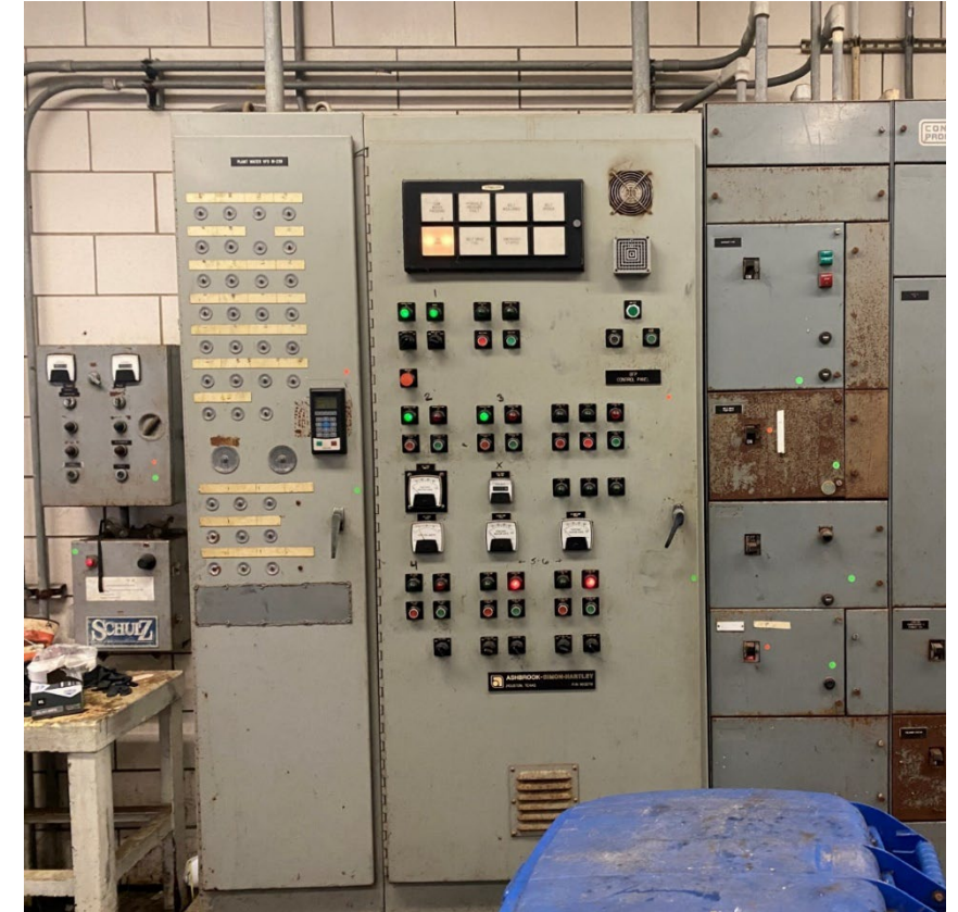
Typical Electrical Panel
