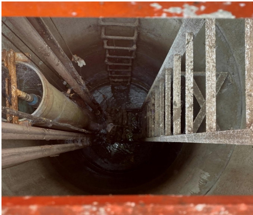
Stony Brook Pump Station: Wet Well & Submersible Pumps.
