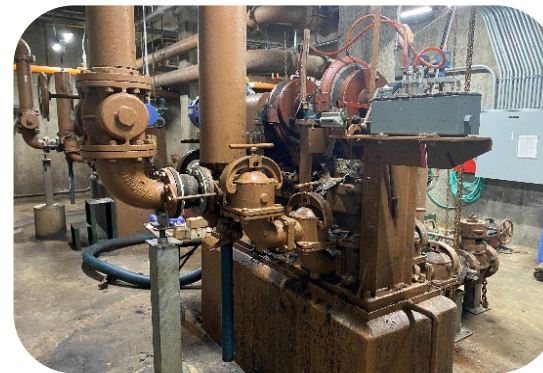
Primary Sludge Pumps
