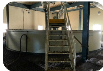
Gravity Thickeners and Sludge Collectors
