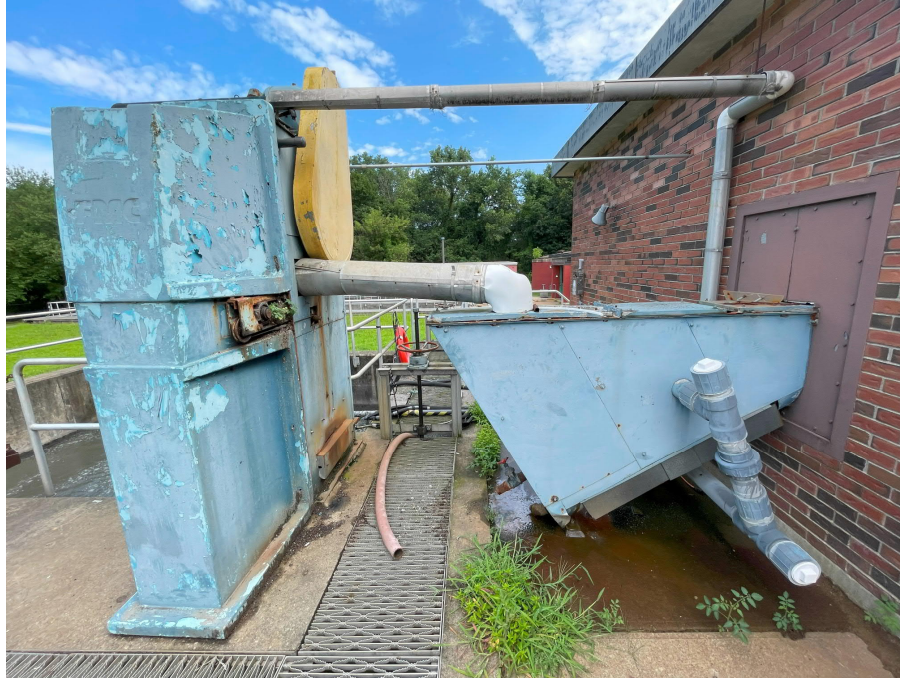
Aerated Grit Facility Equipment: Grit Elevator.
