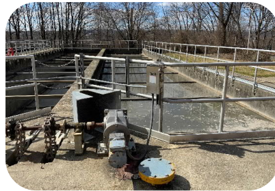
Primary Clarifier Sludge Collectors
