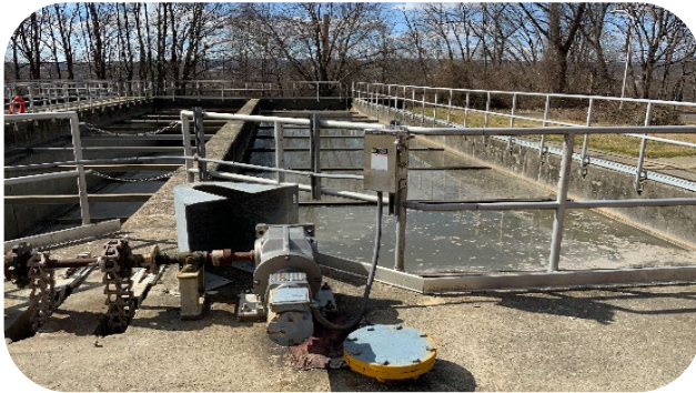
Primary Sludge Collectors
