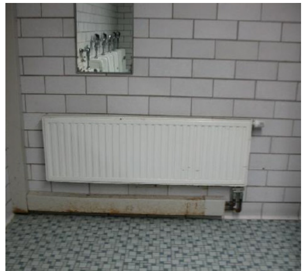
Bathroom radiator with piping cover
