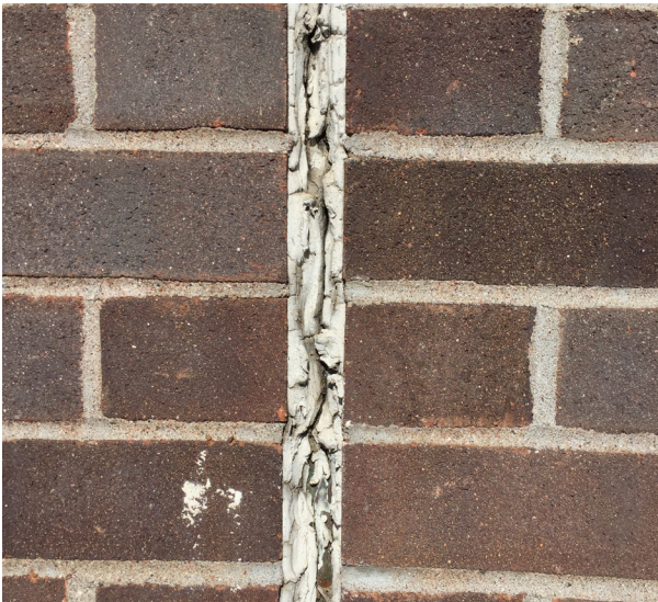
Deteriorated cock joint
