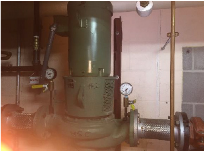
In-line building hot water pump
