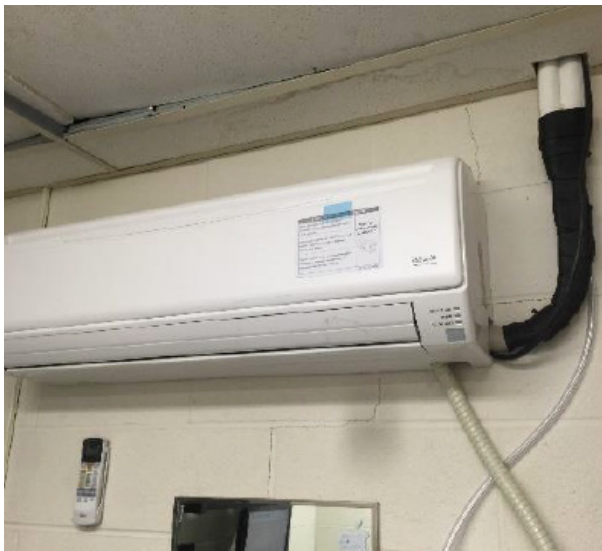
IT Room, ductless air conditioning unit
