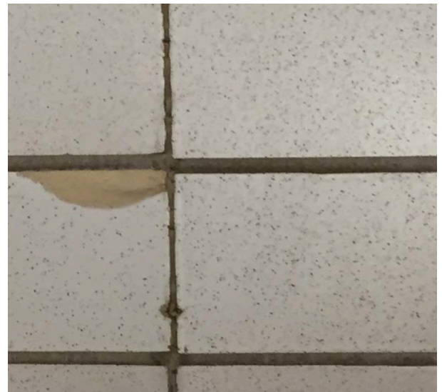
Typical spalling at glazed tile in corridor walls
