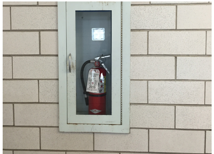
Accessible fire extinguisher
