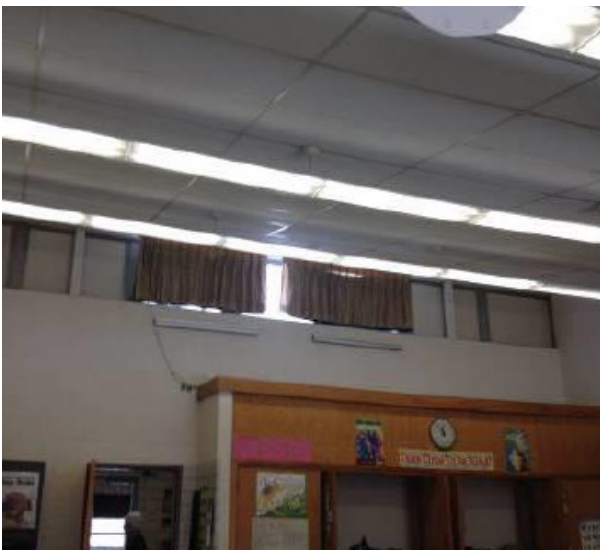
Typical classroom pendant lighting
