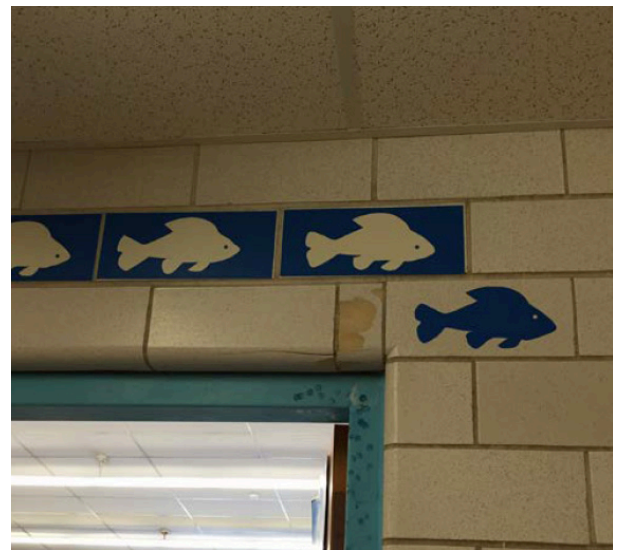
Common spall at corner of door openings
