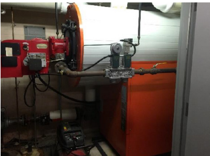
Large Veissman gas-fired boiler
