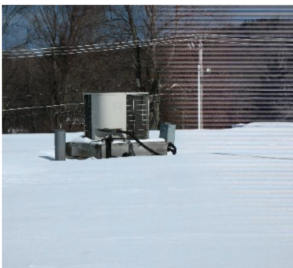
Administration area, condensing unit
