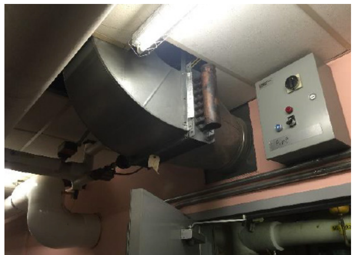
Hot water duct coil for boiler room
