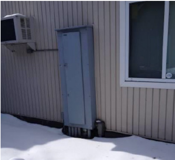
Portable classroom distribution panel
