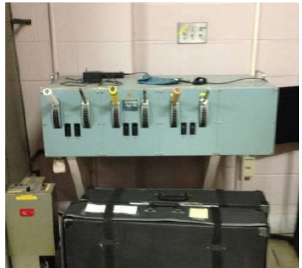
Stage dimming system
