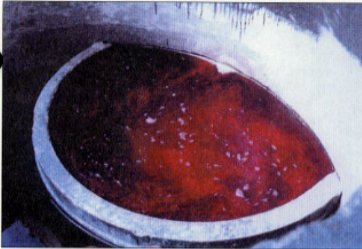
PLATE 4: View of the inlet to the X-Ceptor with flow contained behind the overflow weir at 9l/s. Note the marked difference in colour between the red, oil polluted inflow and the near-clear waters just prior to outlet, having passed through the treatment chamber.
